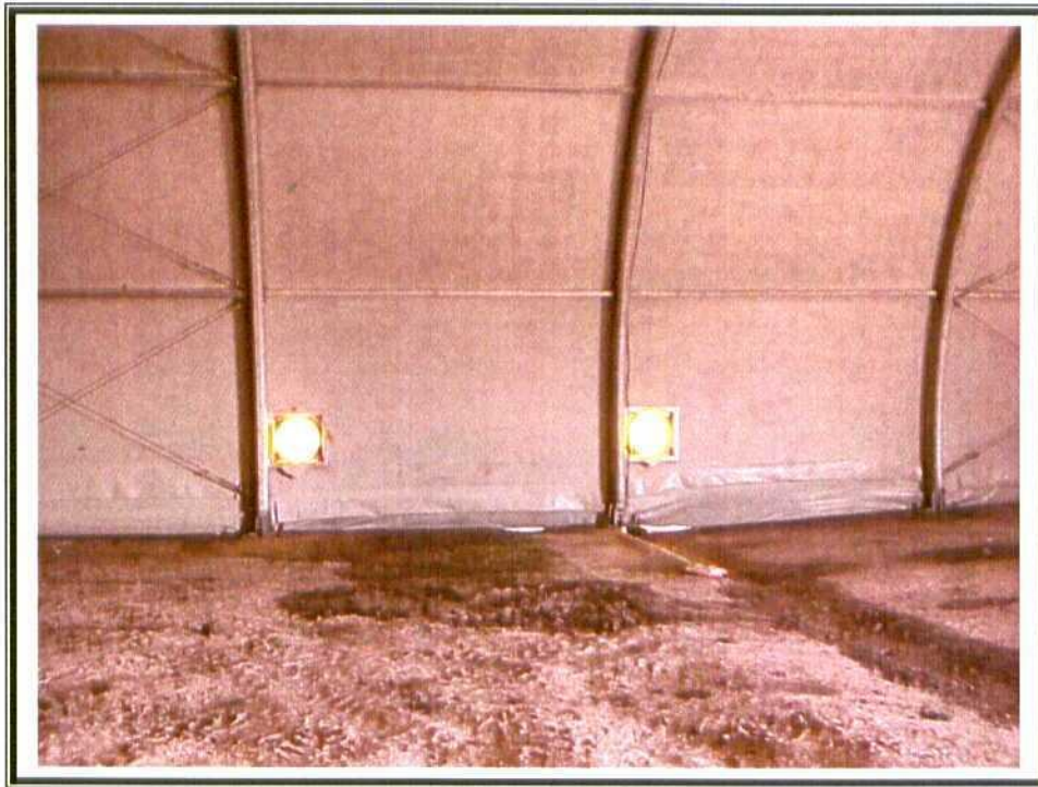
6. Air intake inlets that lead to carbon filtration system.
