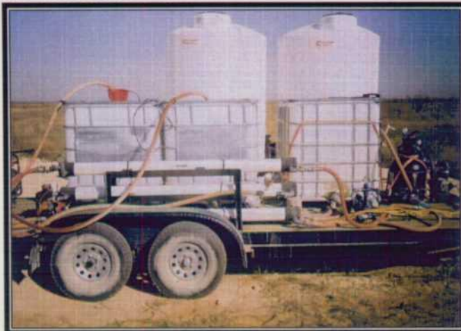
RO Membranes and tanks
