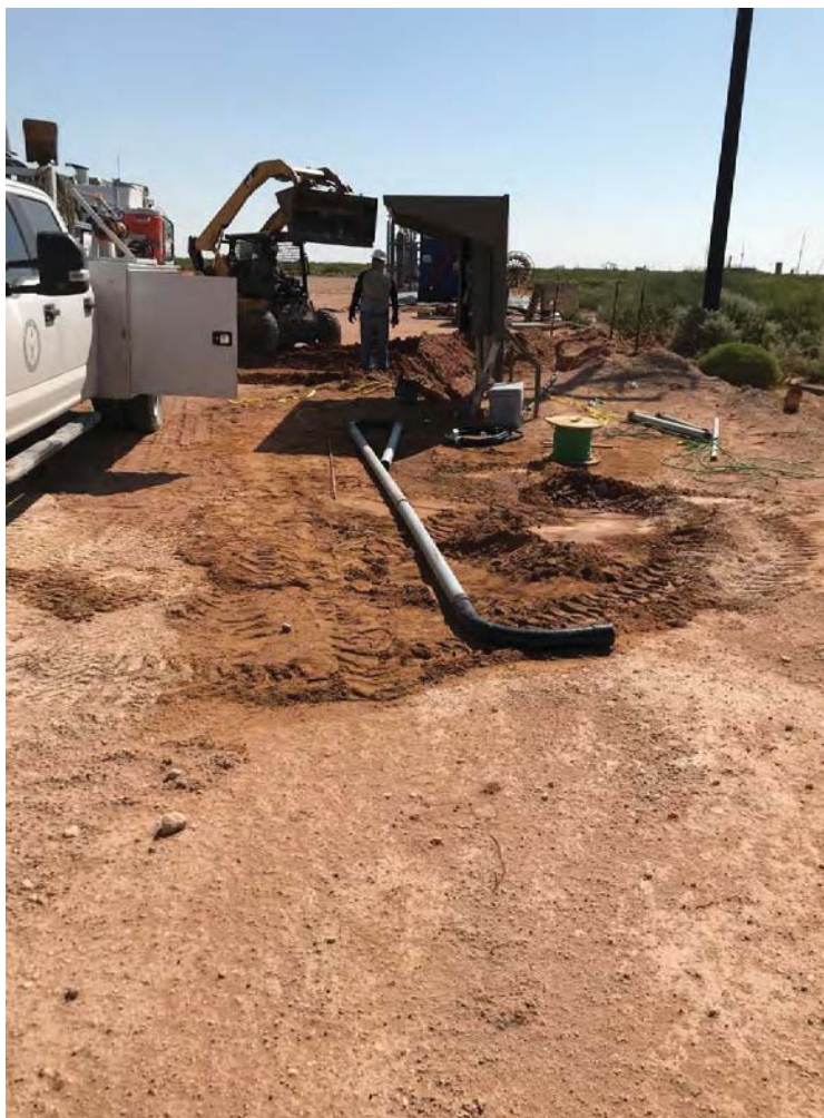
View of the surficial staining facing east. Note the surrounding equipment and utility lines immediately south of the release.
