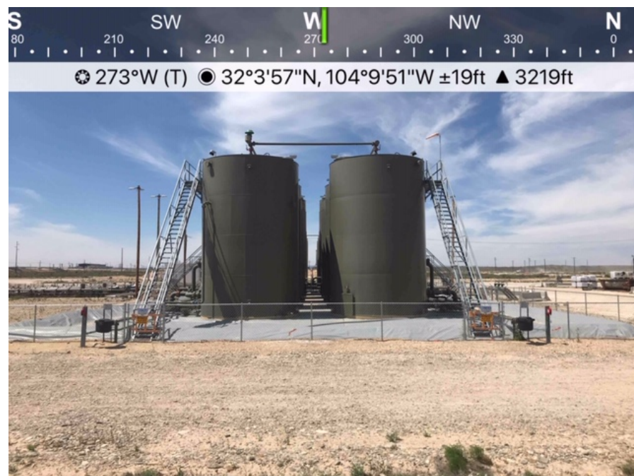
Spill within lined containment viewing west
