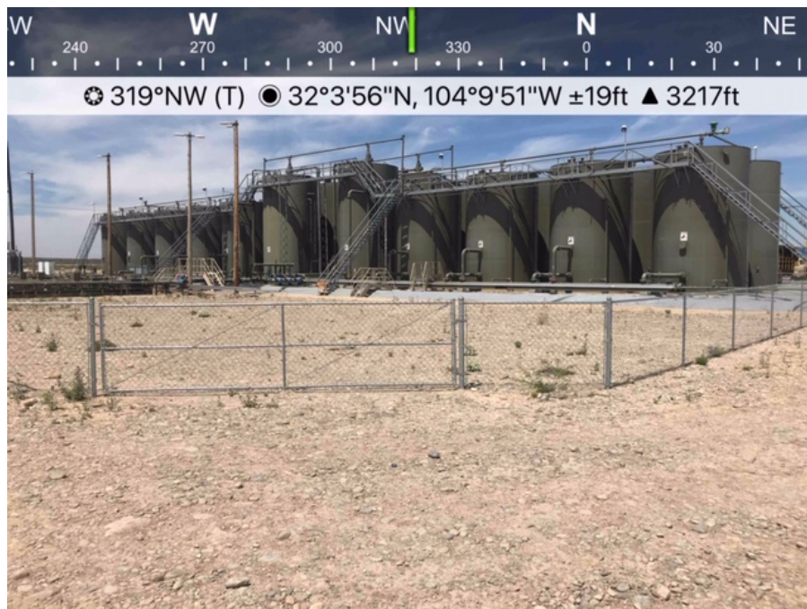
Spill within lined containment viewing northwest
