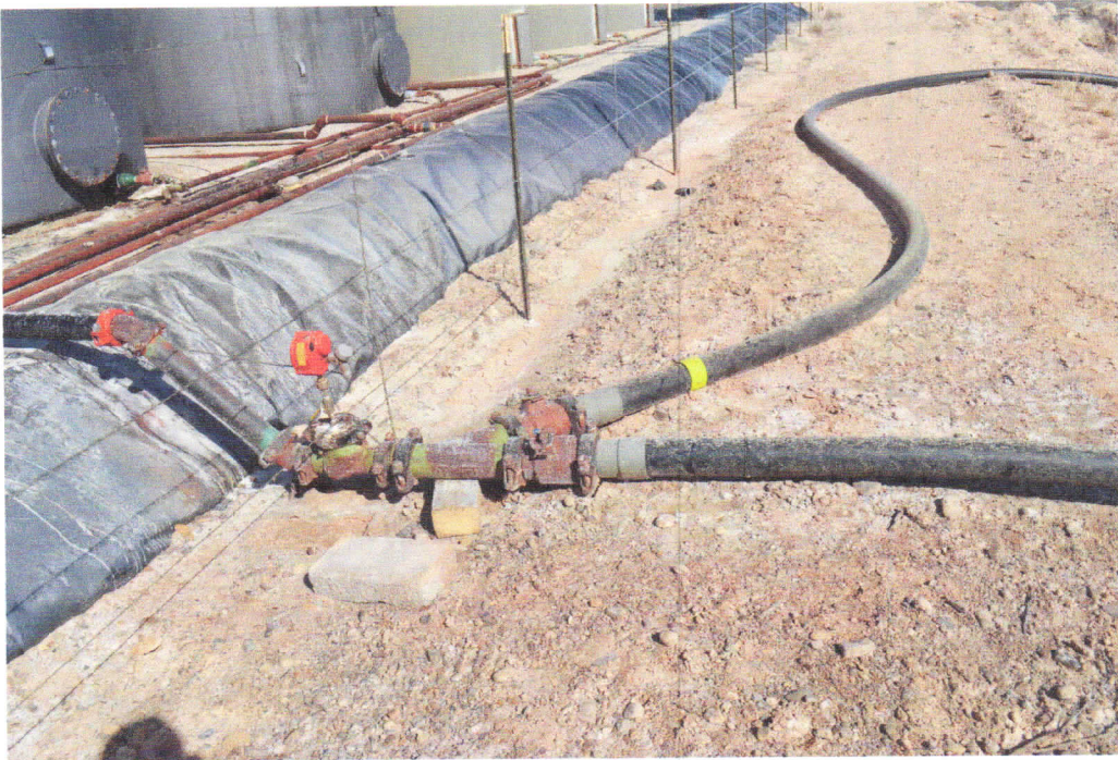
View looking East at area where failure occurred
