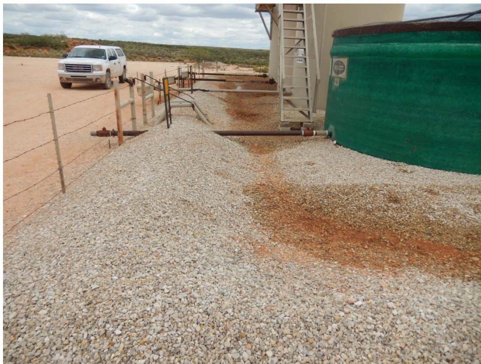
Stained Area Inside Firewall Viewing East, June 1, 2016
