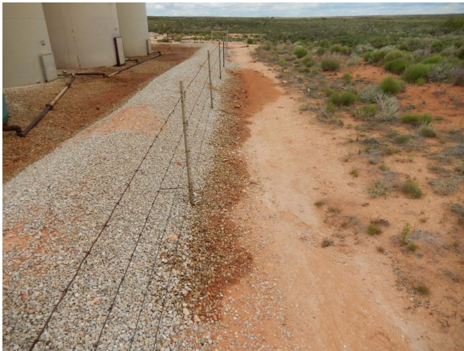
Stained Area Inside and Outside Firewall Viewing West, June 1, 2016
