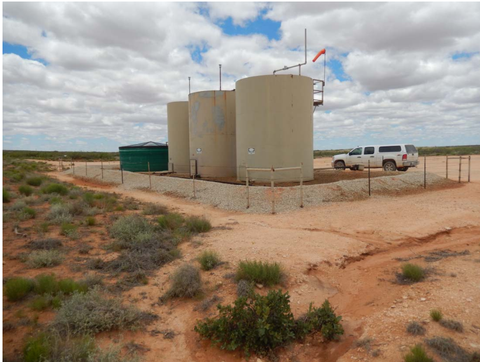
Stained Area Inside and Outside Firewall Viewing Northeast, June 1, 2016
