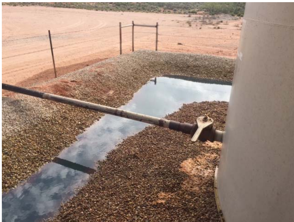
Crude Oil Inside firewall near Northwest Corner (DP-1) Viewing Northeast, May 20, 2016
