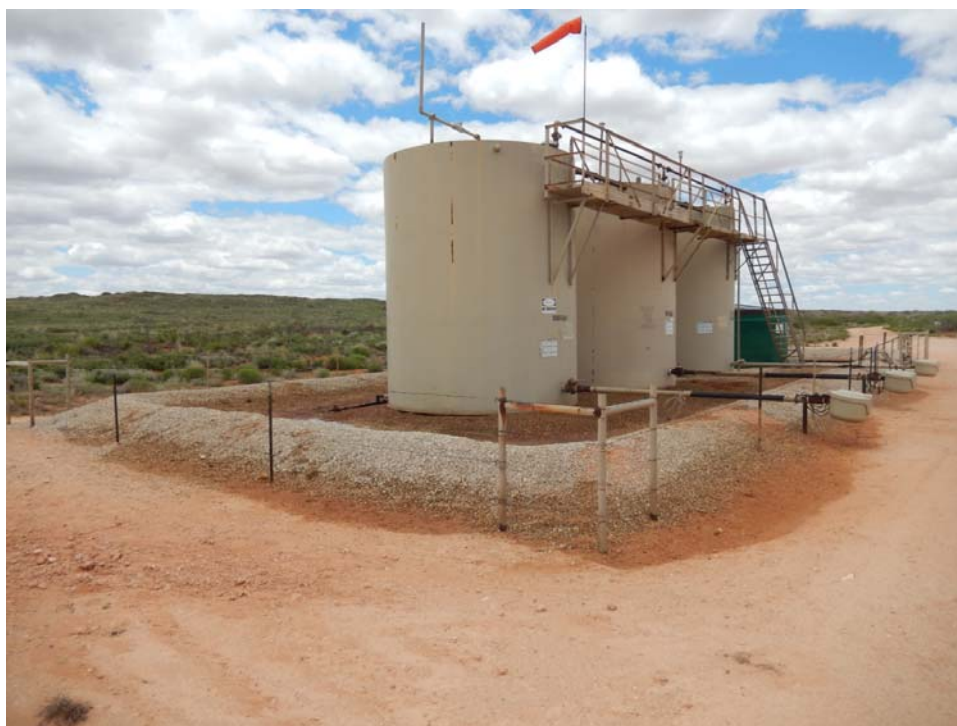
Stained Area Inside and Outside Firewall Viewing Southeast, June 1, 2016
