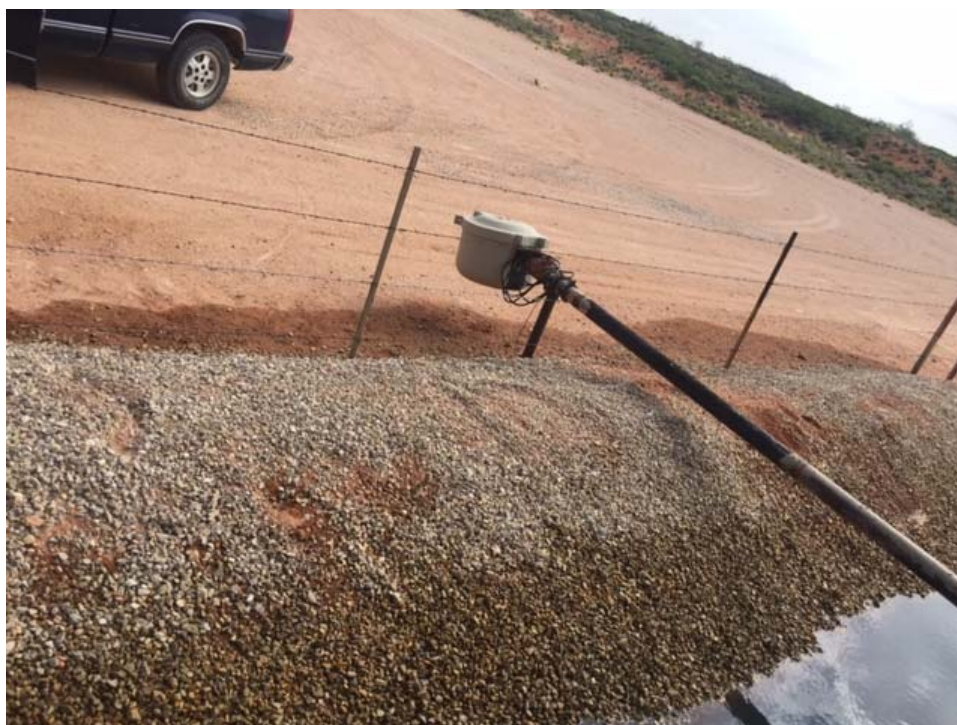
Stained Area Outside Firewall North of Tanks Viewing Northeast, May 30, 2016
