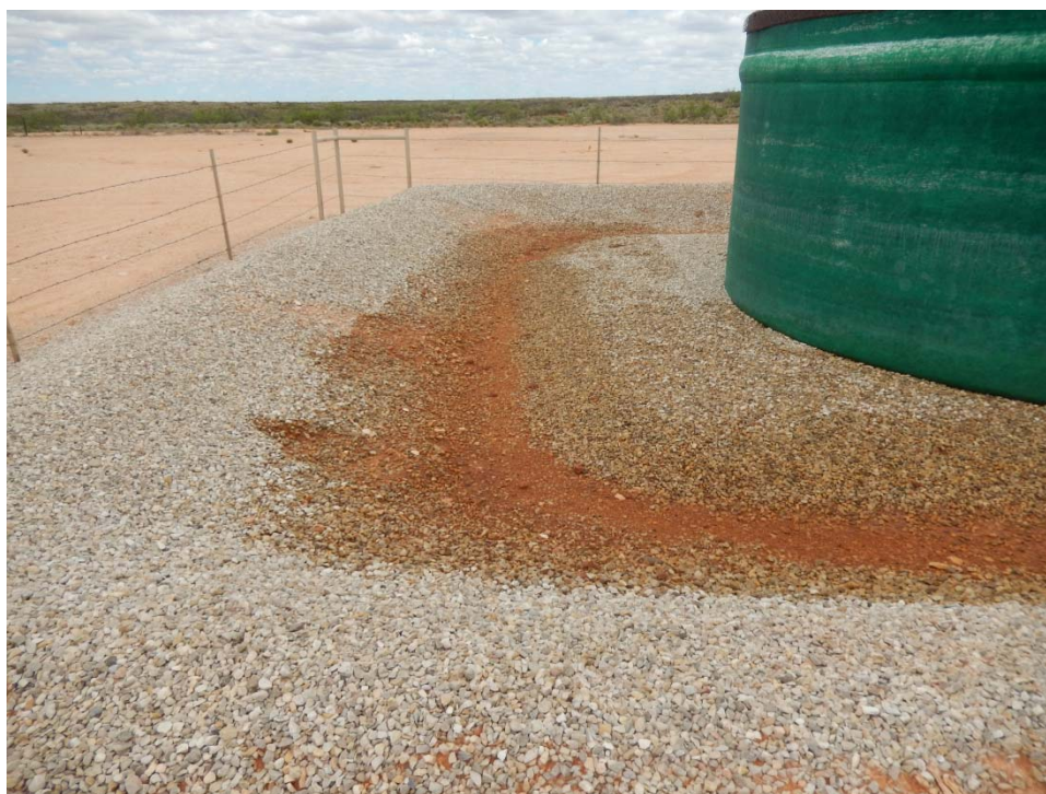
Stained Area Inside Firewall Viewing North, June 1, 2016
