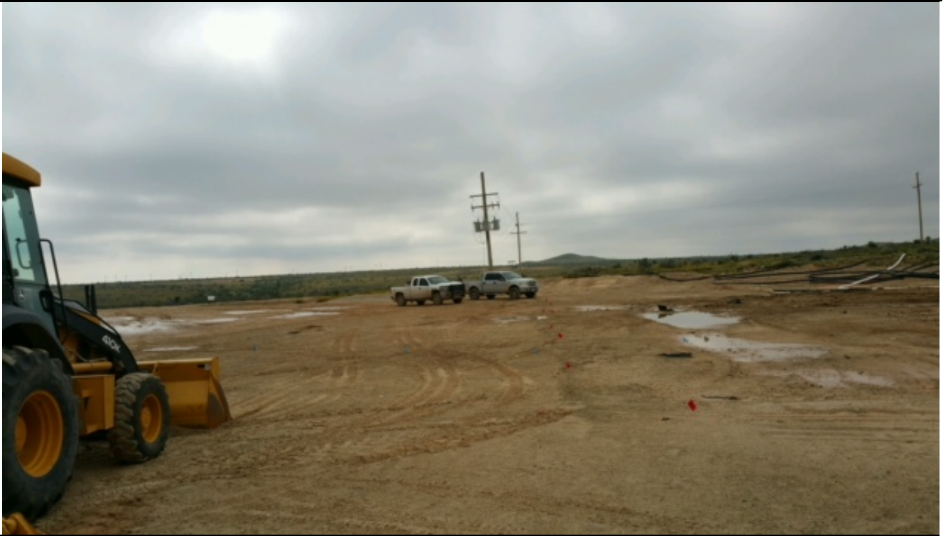
Photo 1: View of portion of the affected production pad, facing south.
