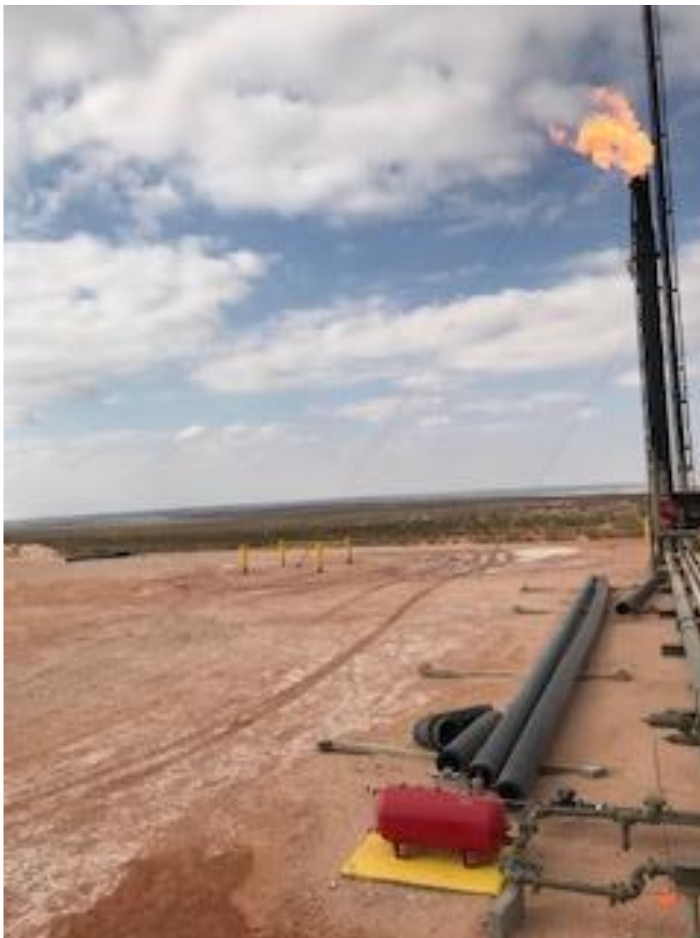
View from the well pad facing the pasture, with the active flare stack on the northern edge of the pad.
