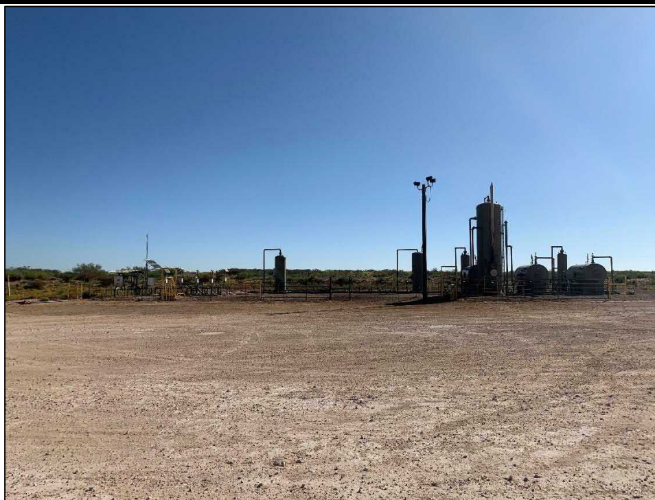
PHOTO 1: View of PLU #387H Heater Treater Facility facing east. 10/17/19
