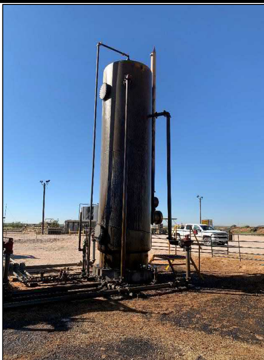
PHOTO 9: View of fluid release source facing south-southwest. 10/17/19
