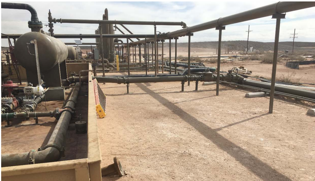
Photograph 1: View of process equipment area.
