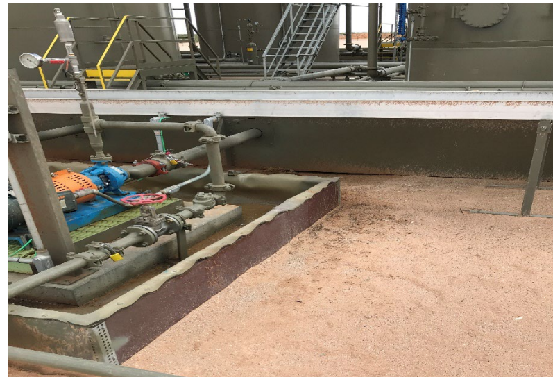
Photograph 4: View of residual soil impacts to west and south of pump.
