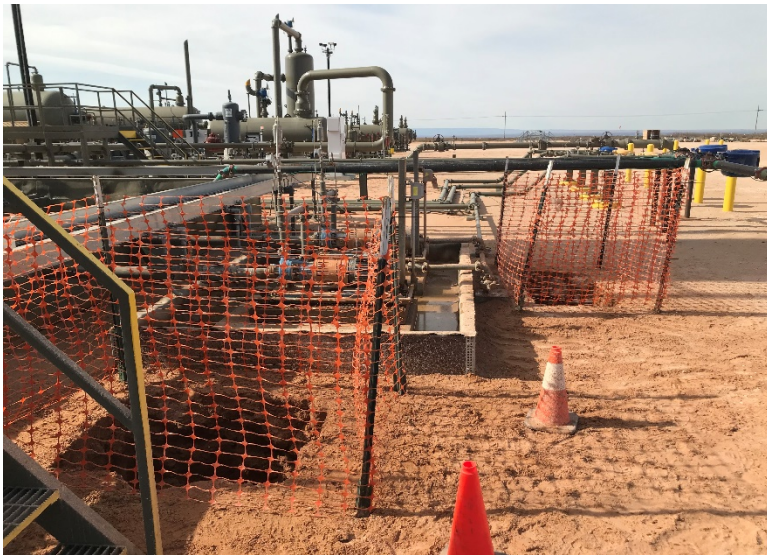
Photograph 3: View production equipment to south and west of release.
