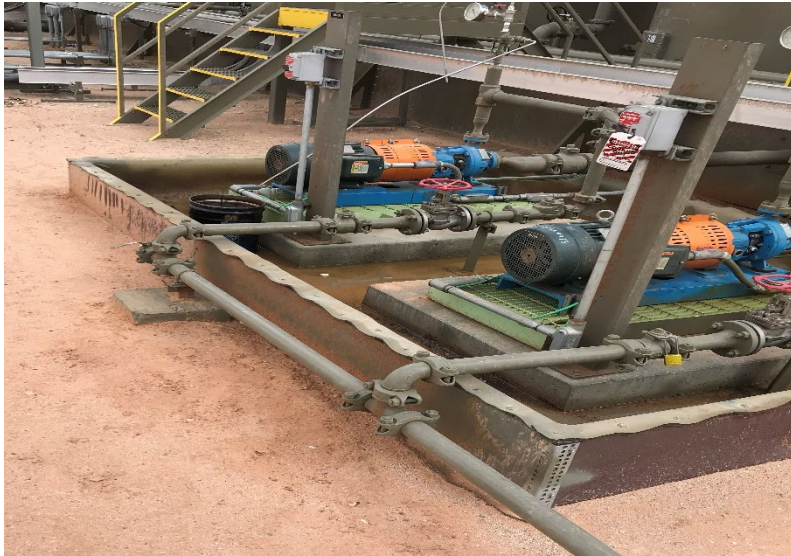
Photograph 1: View of circulating pumps and containment.
