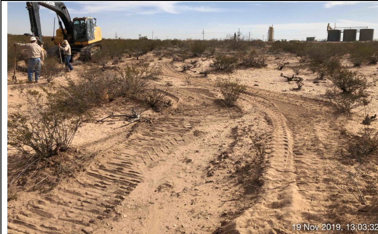
Photo 1: Main body of the affected area viewed to the northwest.
