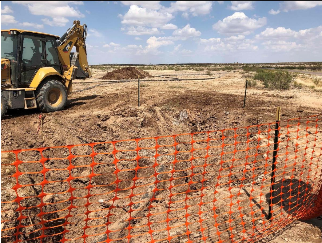
PHOTO 1: View of release origin, facing northeast. 8/14/2019
