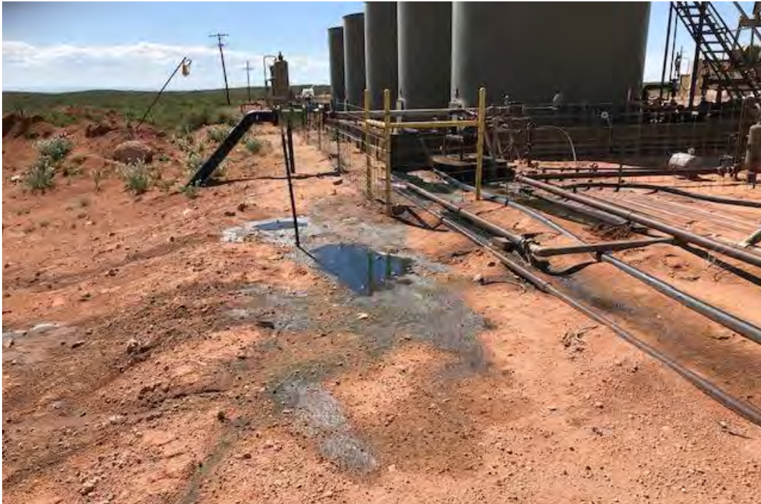
Western view of point of release area on the caliche well pad during site assessment activities.
