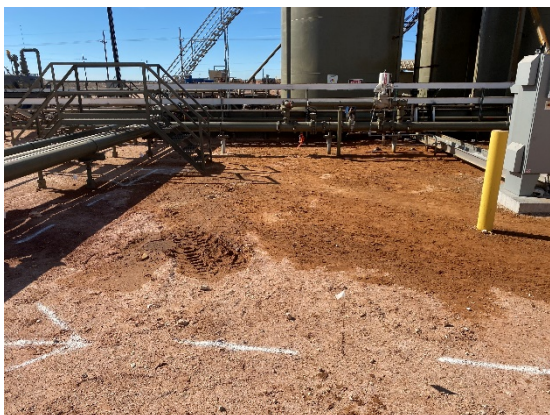
Photograph 1: View of staining on pad between active equipment facing south.
