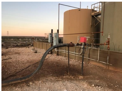
Photograph 11: Point of release west of the tank battery containment.
