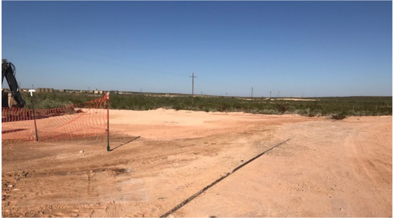
Release footprint on pad surface before excavation– view east toward pasture excavation.
