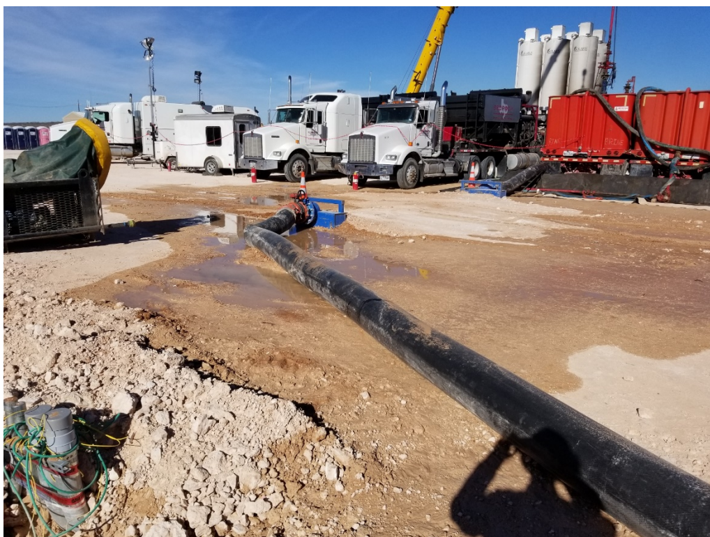
Photograph 1: View of treated water release from west end of pad facing northeast.
