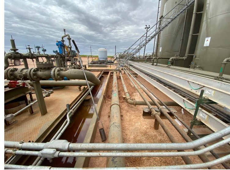
Photograph 2: Western view of staining being addressed near BH01.
