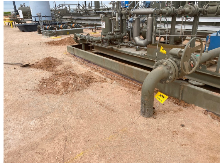
Photograph 8: North western view of staining being addressed near BH04.
