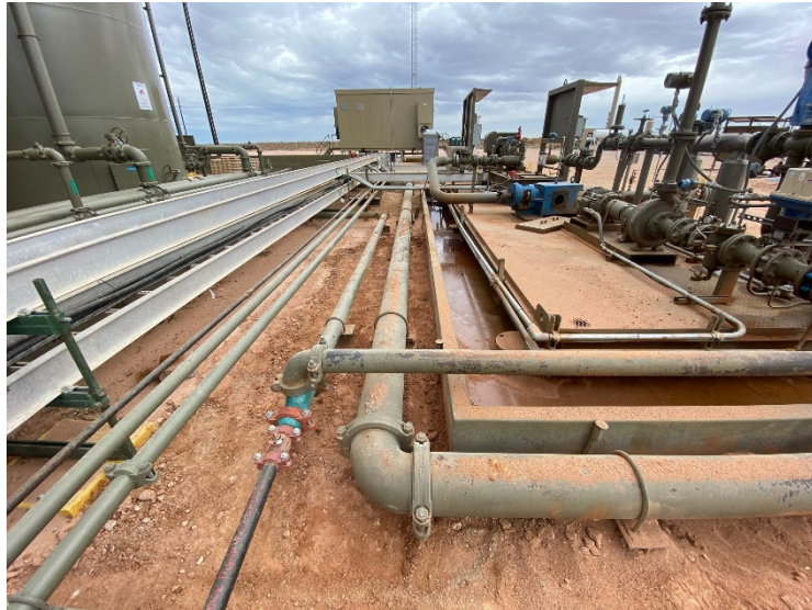
Photograph 5: Eastern view of release after staining is removed.
