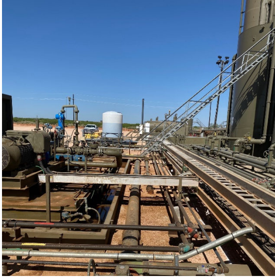
Photograph 1: Western view of visible staining near BH01.
