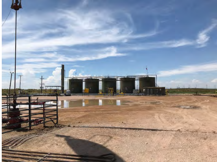
Photograph 1: View of spill on-pad facing west.
