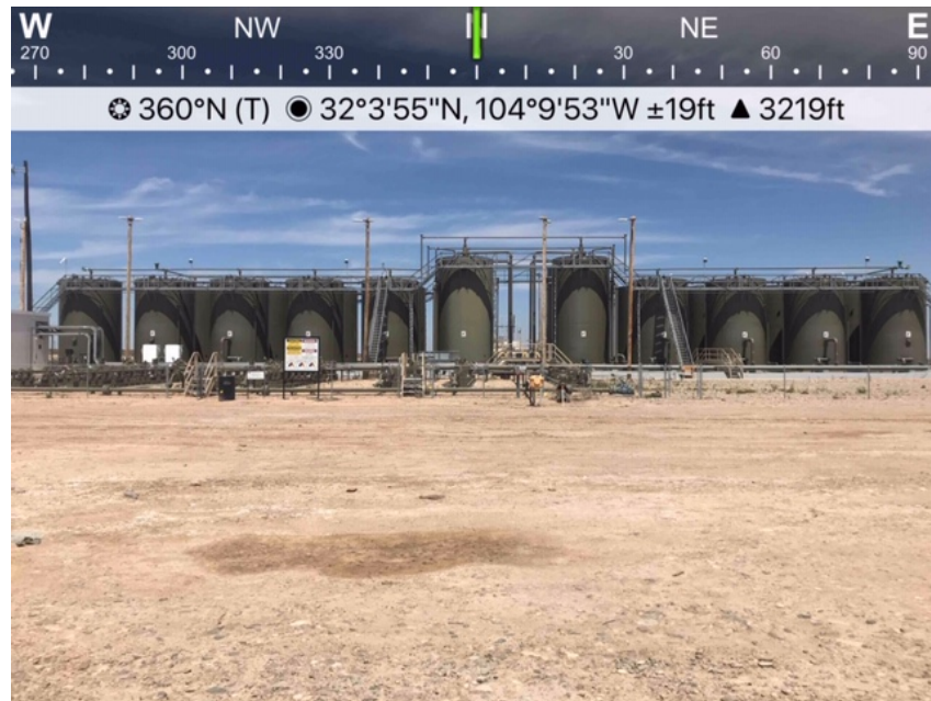
Spill area viewing north
