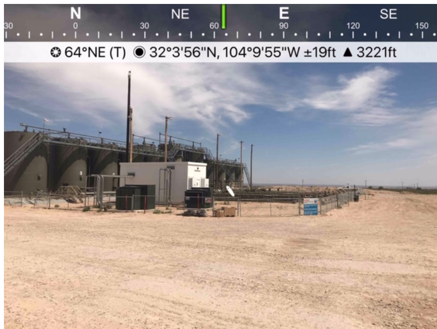
Spill area viewing northeast/east
