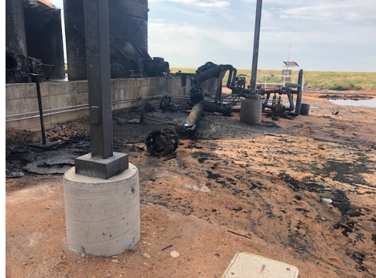
Photograph 2: Damage to tanks and liner due to fire.
