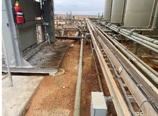
Photograph 1: View of release to the south of the tank battery facing west.
