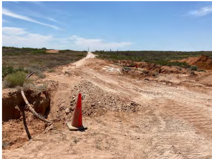
Photograph 4: Western view of road scrape near release point in pasture.
