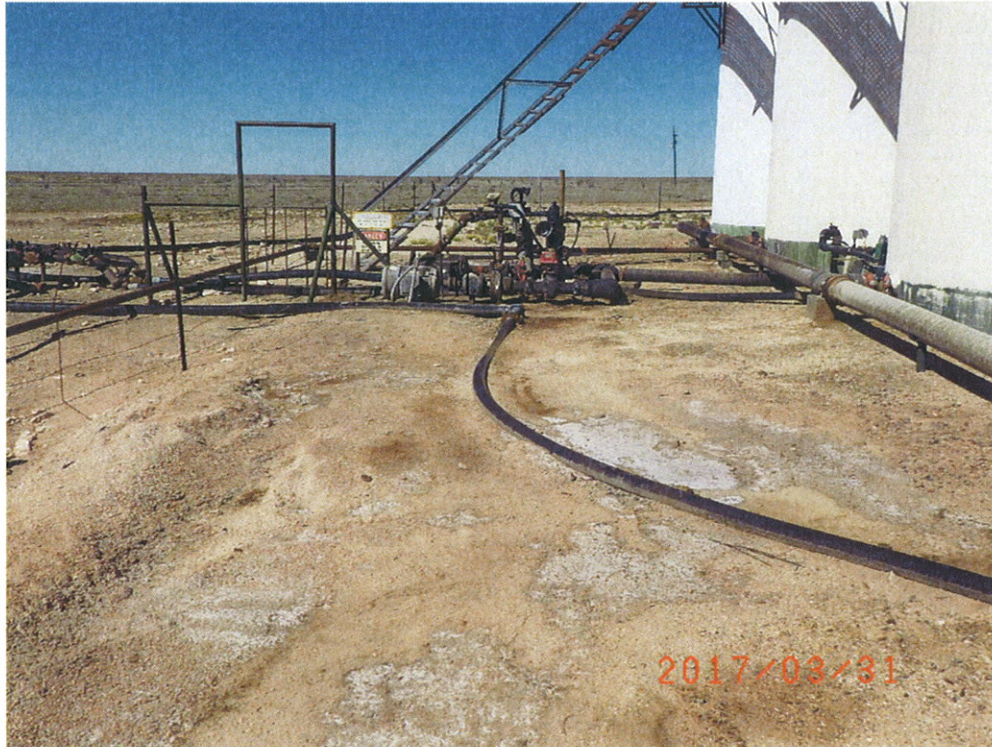
Spill Area South of Battery Viewing West
