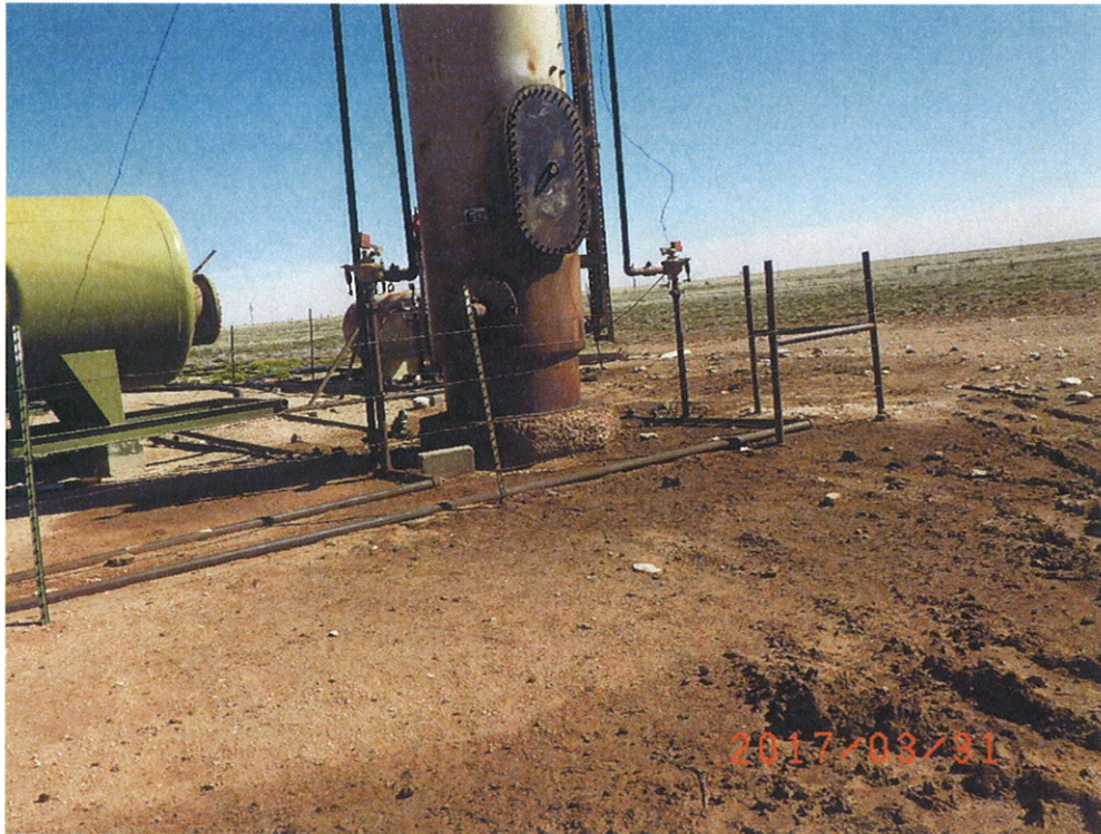
Spill at Separator Viewing Northeast
