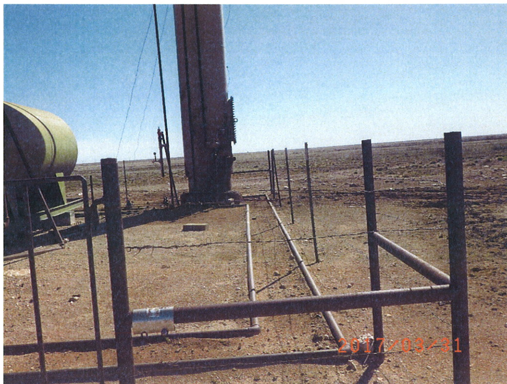
Spill at Separator Viewing East
