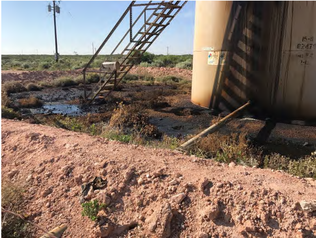
Red Tank 24 Fed 1 & 2 CTB – Release (Looking Southeast)
