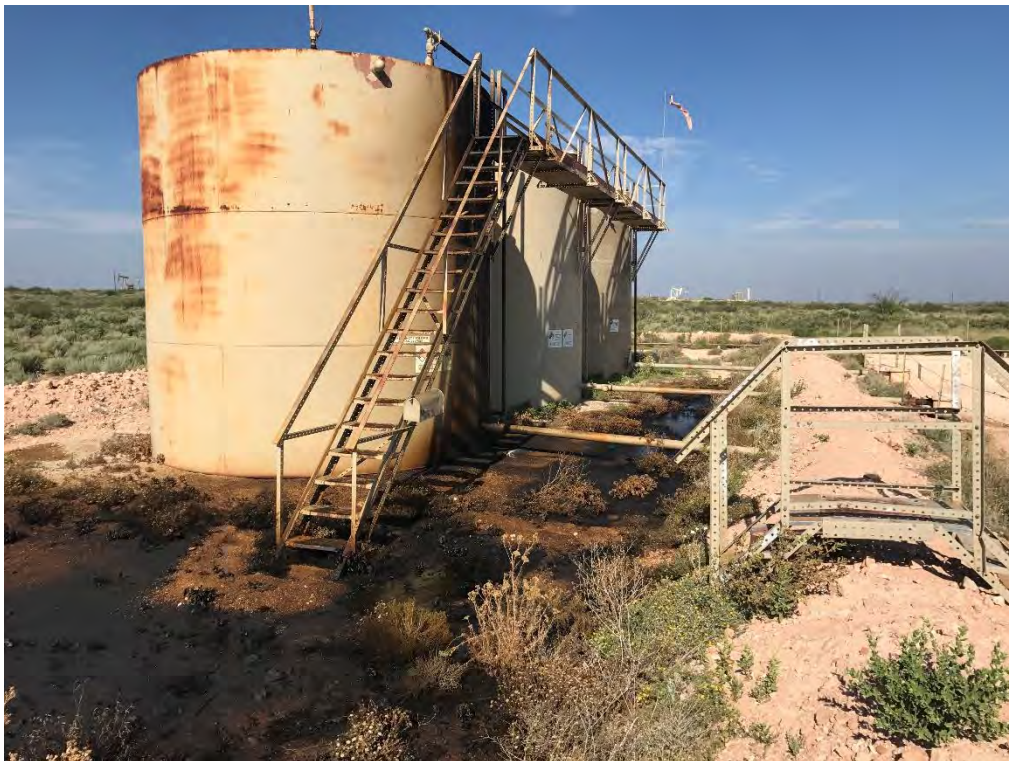
Red Tank 24 Fed 1 & 2 CTB - Release (Looking West-Southwest)
