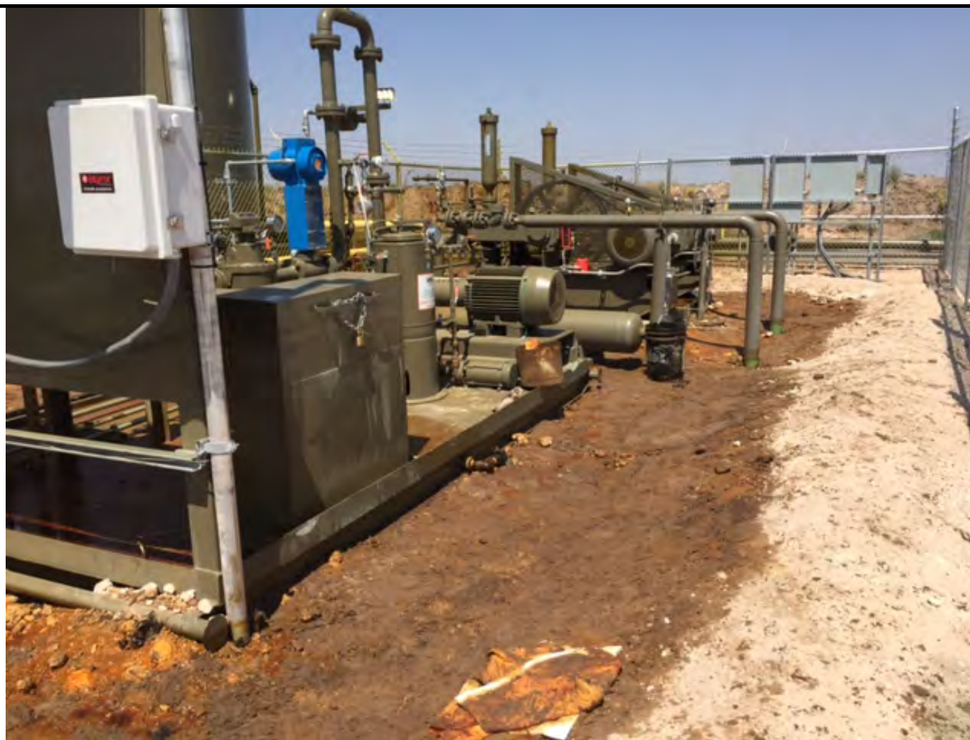
Photo 2: View of surface staining from the initial release, facing northwest.
