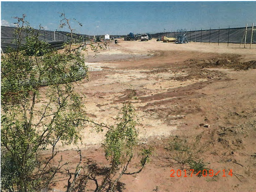
West End of Spill Viewing East
