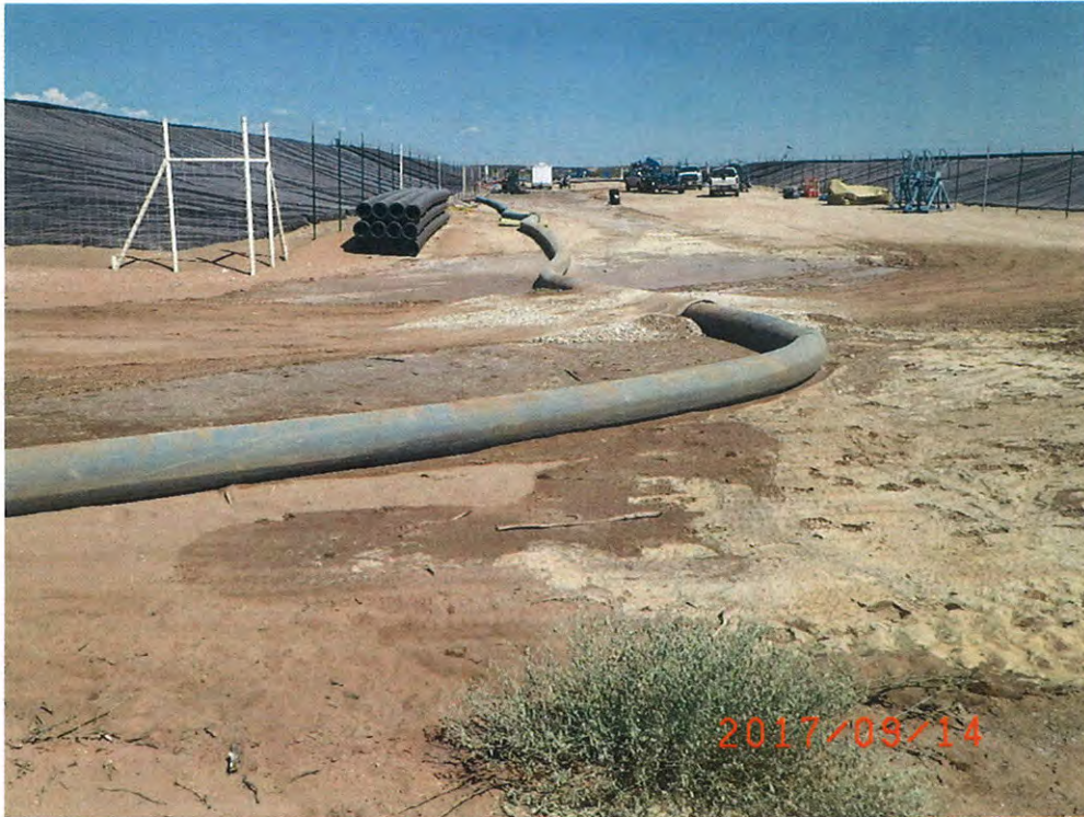
West End of Spill Viewing East
