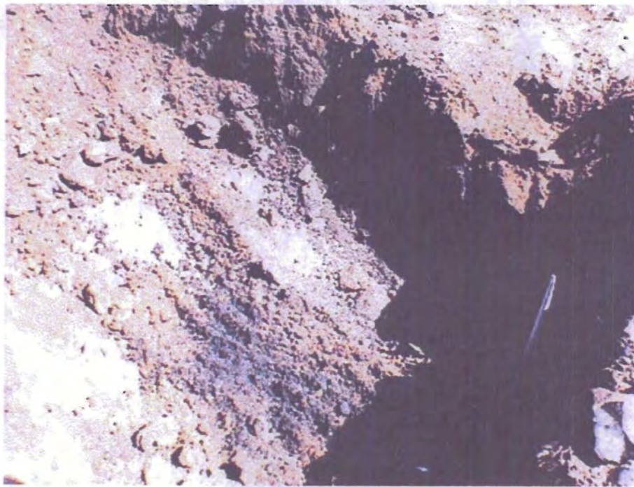
Chevron #214 Leak Site - Excavated Leak Area
