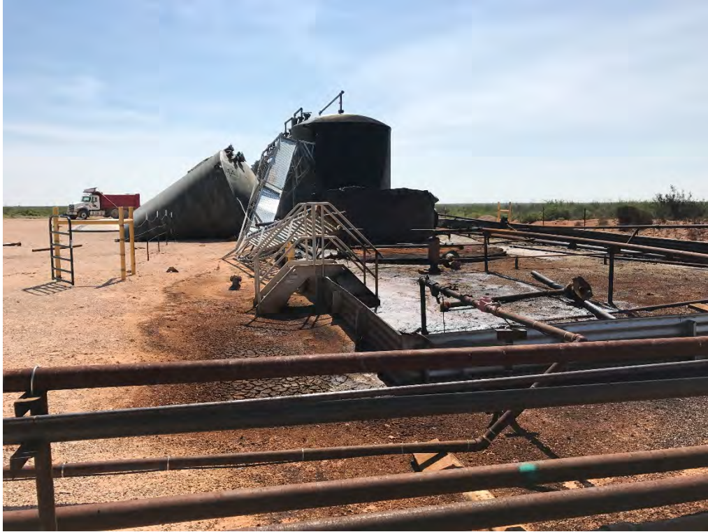
Madera 35 Federal #1H CTB – August 2017 Release (Looking East-Southeast)
