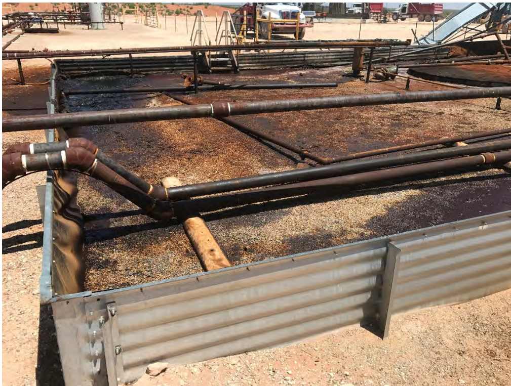
Madera 35 Federal #1H CTB – August 2017 Release (Looking North-Northeast)
