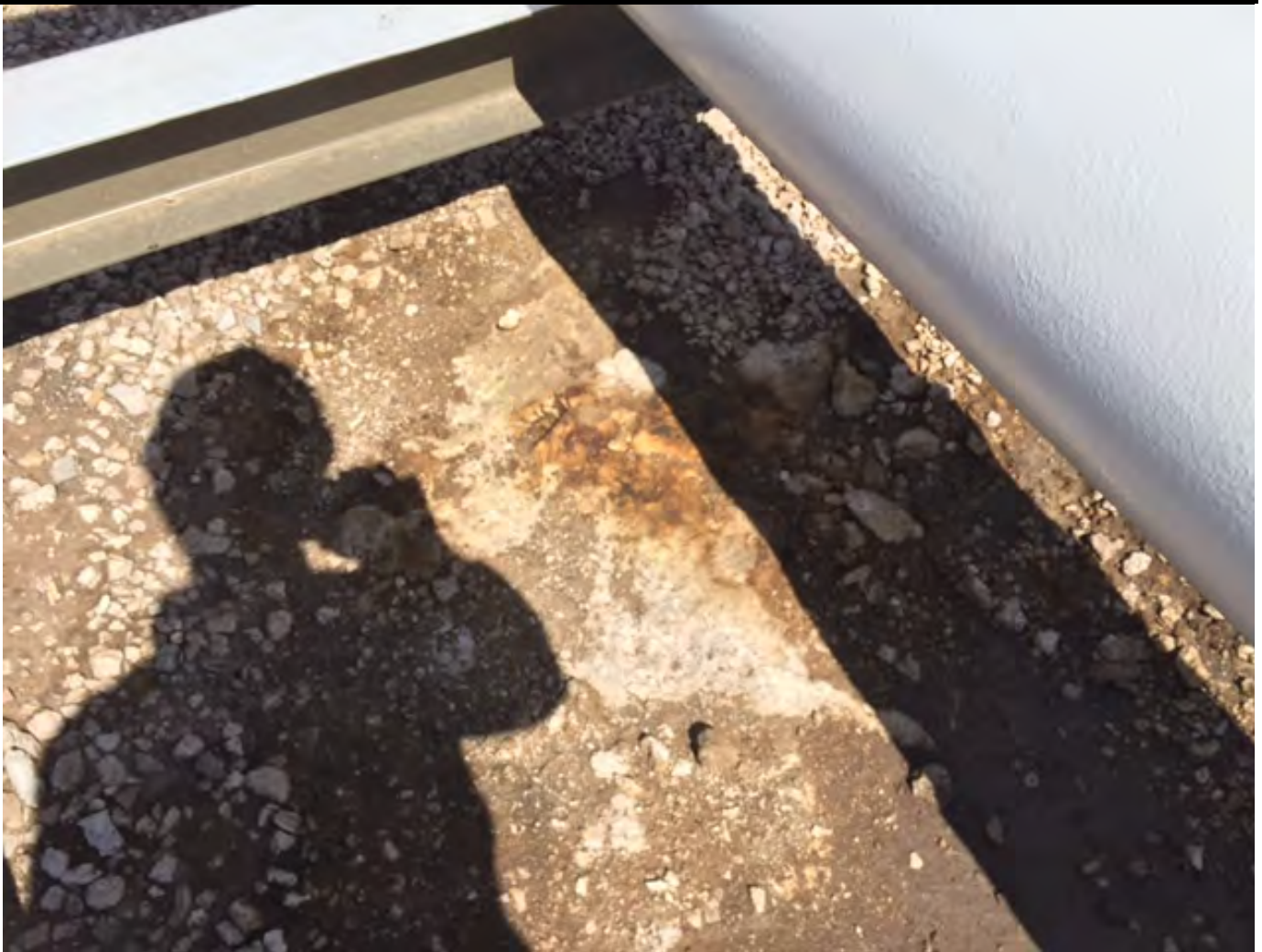
Photo 5: View of the affected area characterized by soil sample FL-2 @ 6" (In-Situ).
