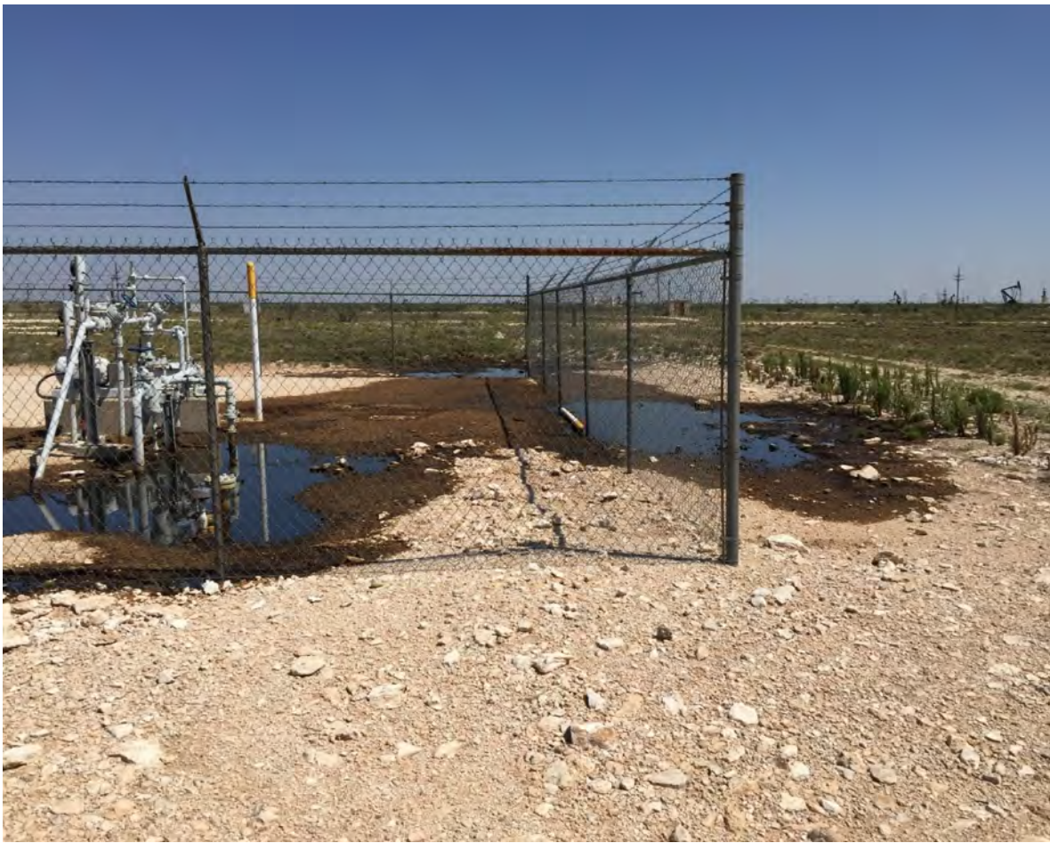
Photo 1: Crude release at pipeline pumping unit. Looking North. August 4, 2018.
