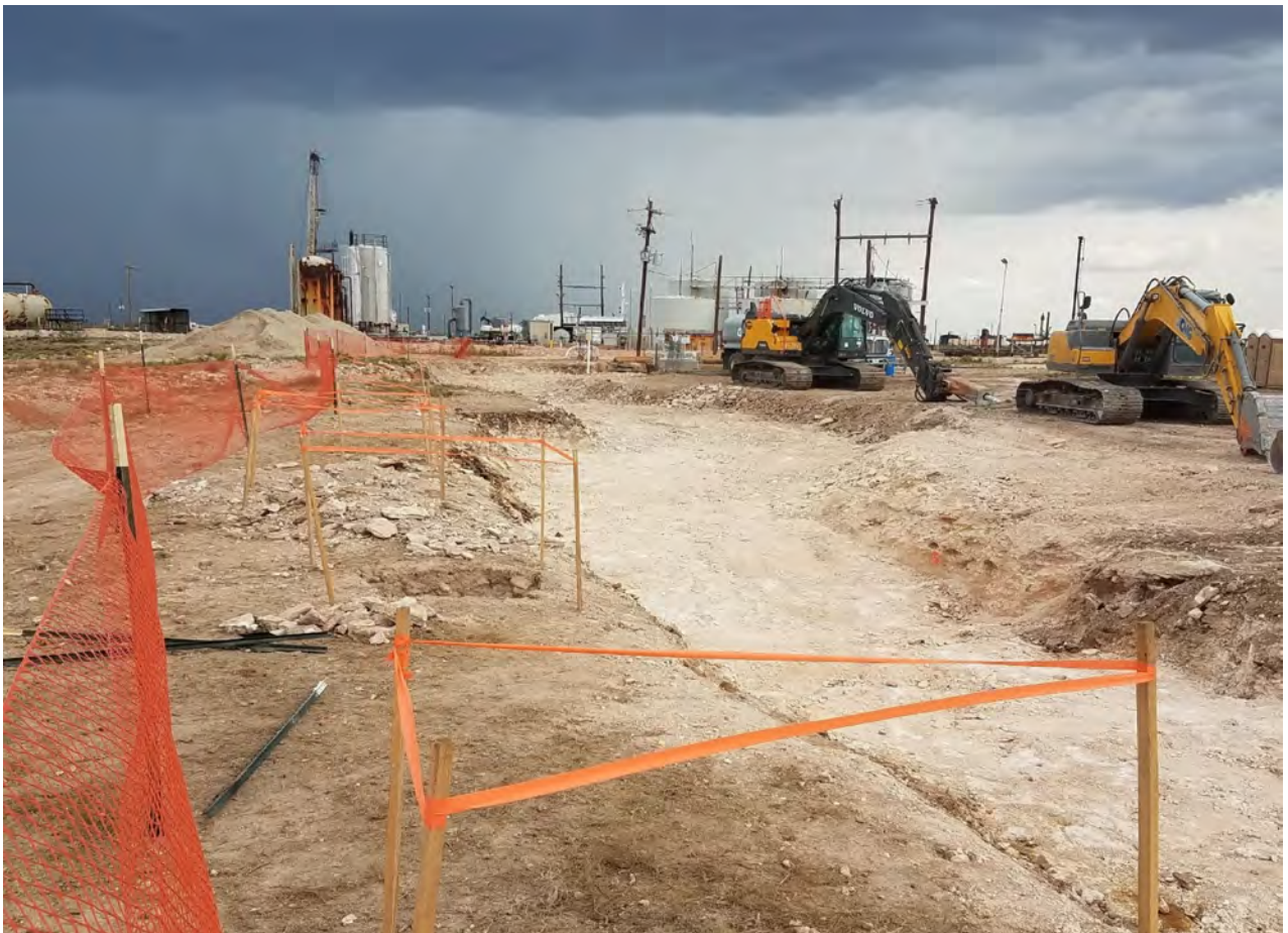
Photo 4: Pipeline potholes east of excavation. Photo looking South towards sump/release point. August 10, 2018.
