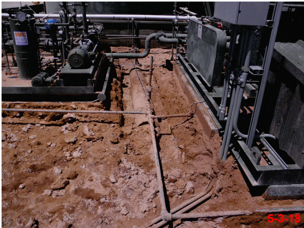
Photo 12 – View of hydrovac activity around LACT Unit equipment facing north
