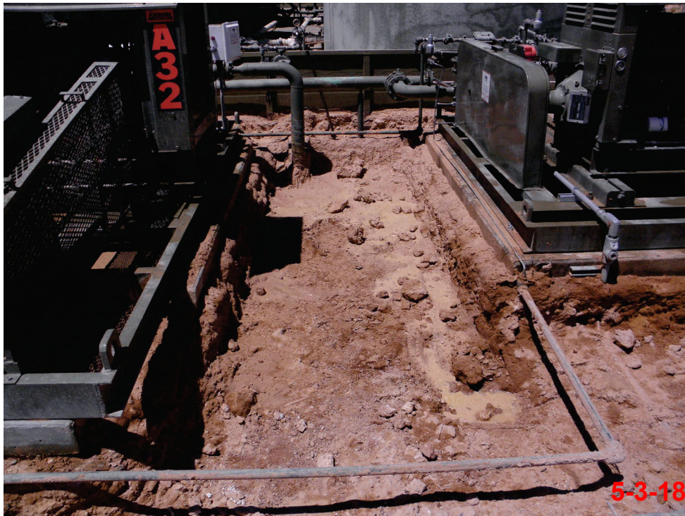
Photo 13 – View of hydrovac activity around LACT unit equipment facing north
