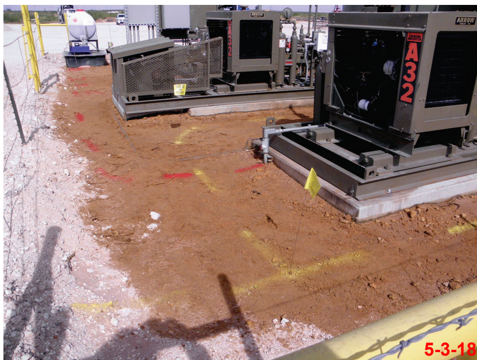
Photo 5 – View of impacted soil along southern edge of LACT Unit facing west
