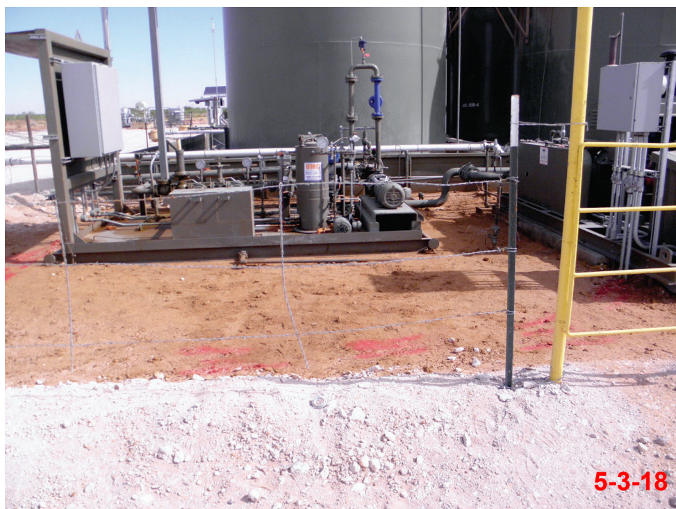
Photo 7 – View of impacted soil around LACT Unit equipment facing north
