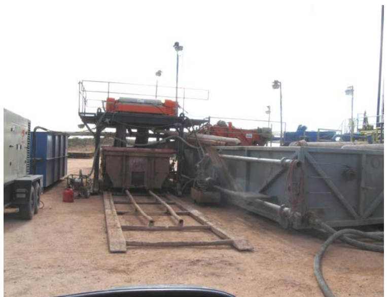
Above: Centrifugal Closed Loop System
